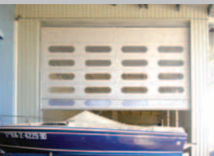
High speed door in a cabin.
