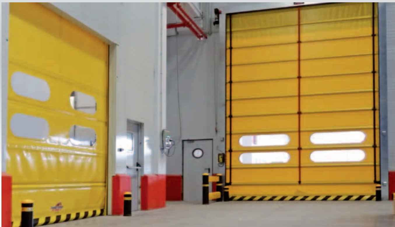
Instant Pass® BASIC at logistic warehouse.
