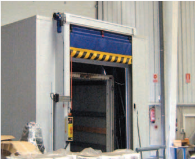
High speed door with loading bay enclosure.
