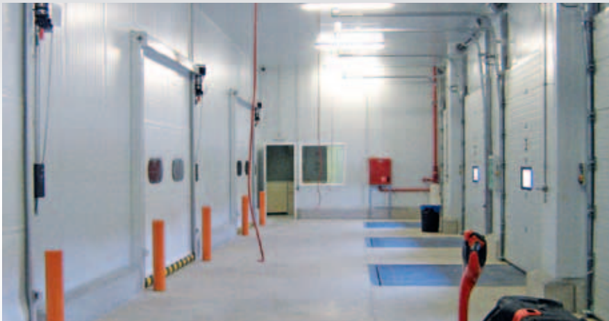
Instant Roll® ECO in freezing logistic center.
