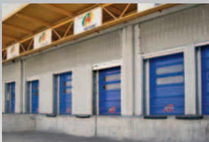
High speed door in loading bays.
