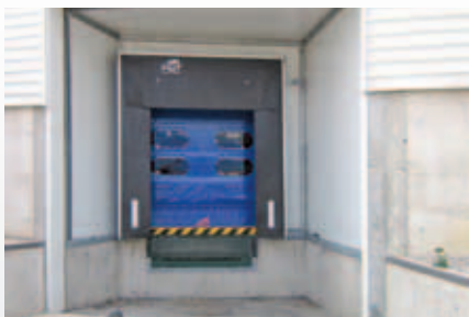
High speed door in loading bay.
