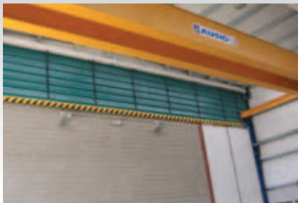
High speed door, gantry crane.
