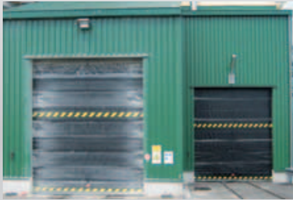
High speed door in Atex area (dust).
